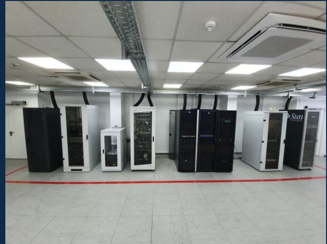
Data center in CIS UoM
